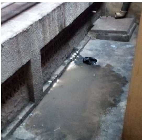
Plate 3: Clogged Drainage in Hostel due to Improper Disposals of PET bottles
